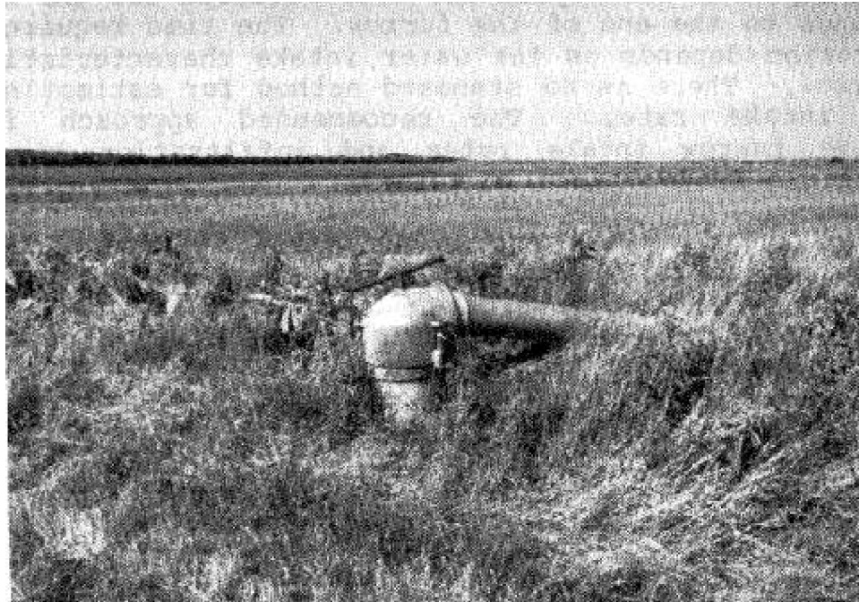
FIGURE E-2 ALUMINUM HYDRANT AND GATED PIPE AT SWEETWATER, TEXAS
